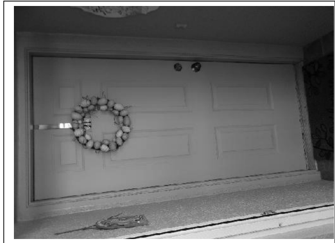
OPENING PROTECTION – Many of the in-swing unit entry doors are not rated or protected
