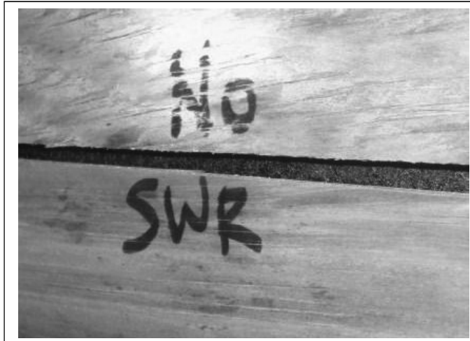
SECONDARY WATER RESISTANCE – Is not installed
